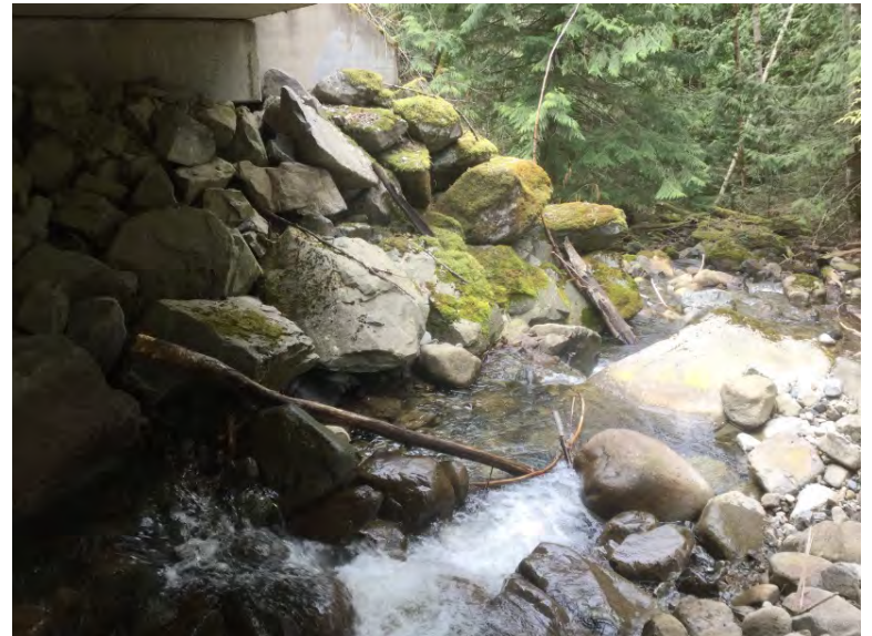
Downstream left bank, steep riprap but appears stable
