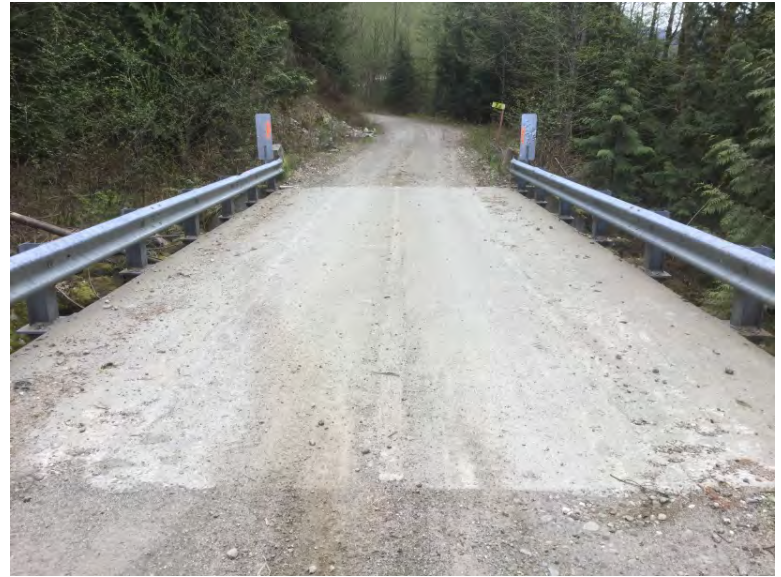
Deck, minor track damage
