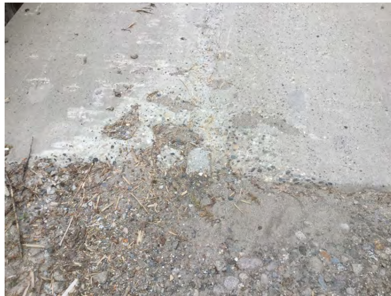
Damage to top of slabs due to tacked machinery
